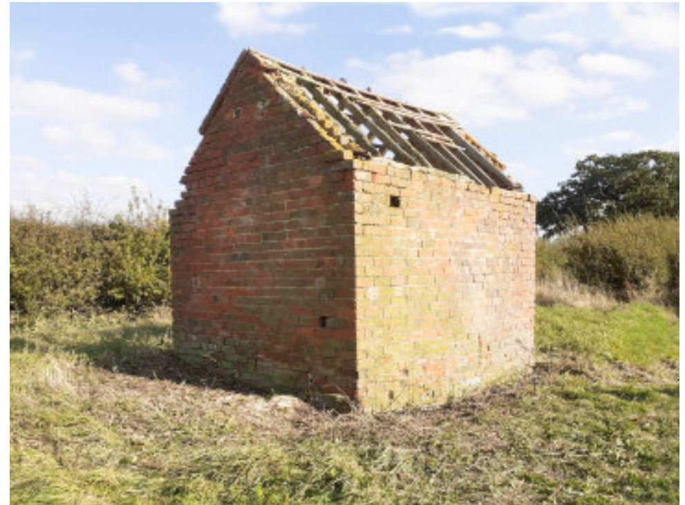
The weigh house (left) before work started and after (above) now ready for restoration works
