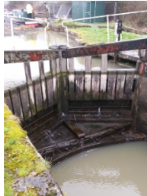
View of Lock 18 showing barely a trickle of water leaking (11 Mar)
