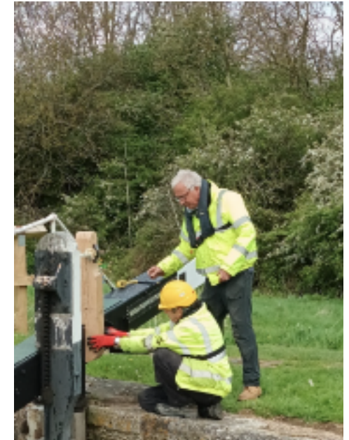
Volunteers Nick & Stephen installing a winding post (crafted by Nick) for Lock 16 (29 Apr)
