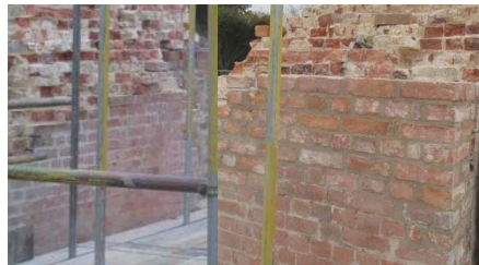
CRT Trainees rebuild part of the corner post using reclaimed bricks and lime mortar
