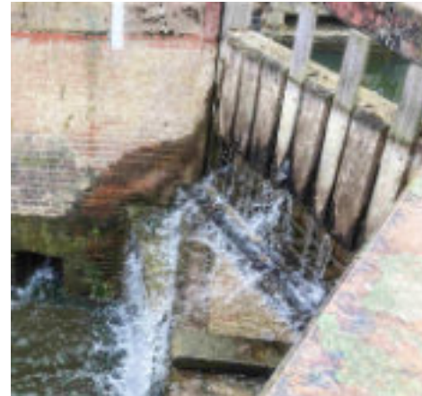
Leaking nearside paddle at Lock 18 (10 August 24)
