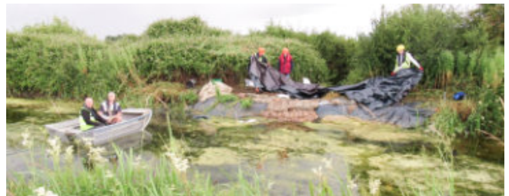
Today's task was to seal the Culvert 12 leak where a temporary fix had collapsed again causing a huge loss of water (6 July 24)
